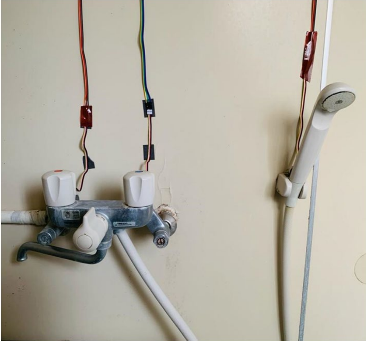
Figure 26. Water taps and hand shower wiring overview
