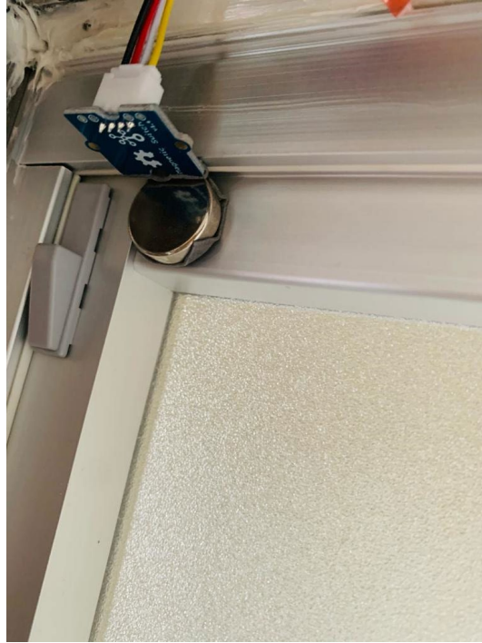
Figure 22. Bathroom Door Sensor (Door Closed - Status1)
