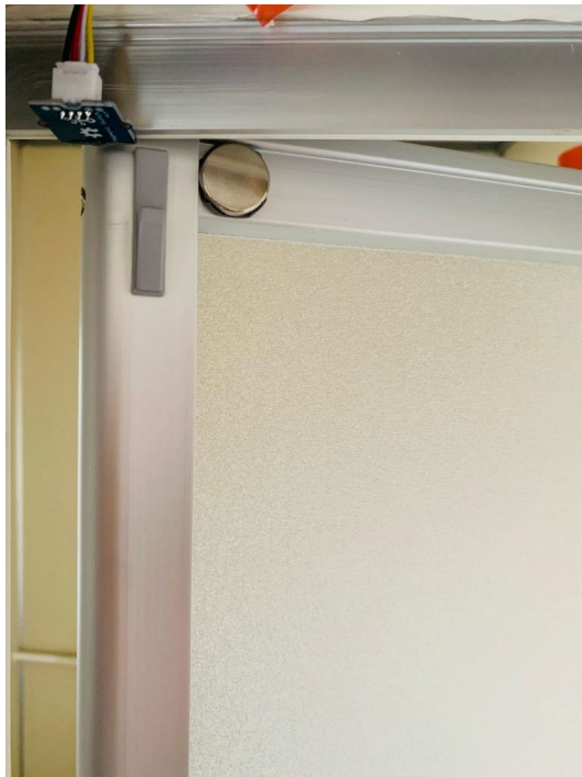
Figure 23. Bathroom Door Sensor (Door Opened - Status 0)
