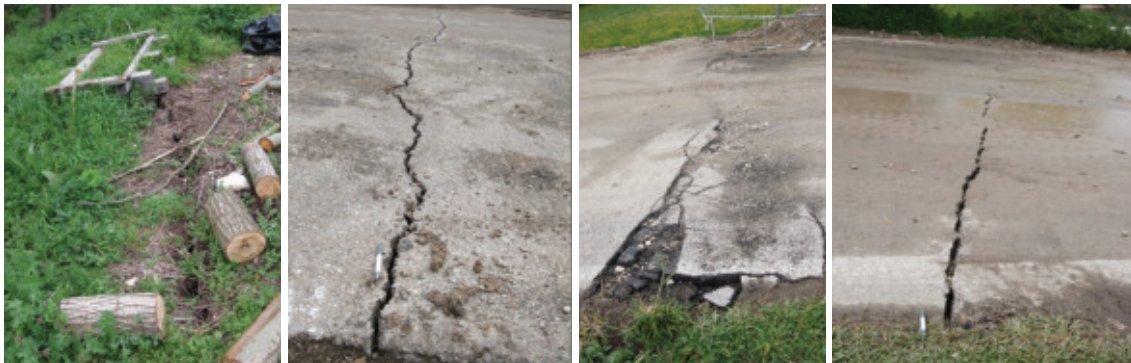
Figure 17. Views of cracking.
