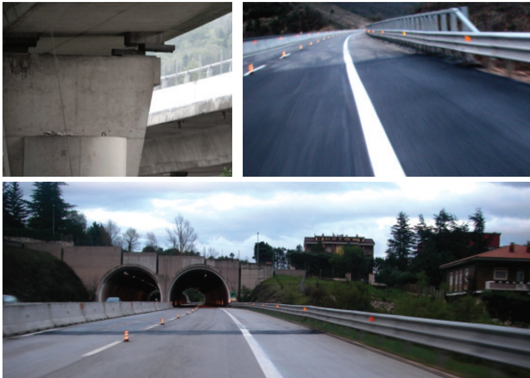
Figure 39. Damage to A24 expressway.
