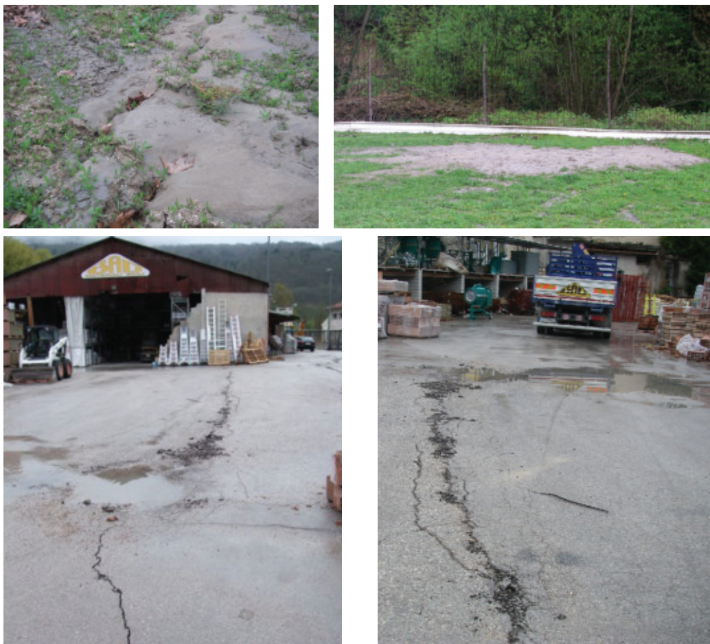
Figure 31. Ground liquefaction and lateral spreading induced damage and ground settlement at the depot yard in Martini district.
