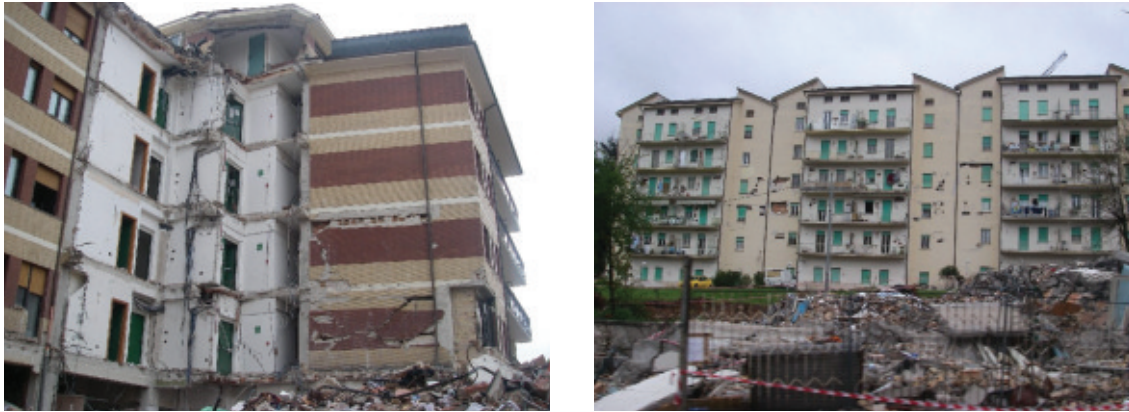
Figure 37. Examples of heavily damaged or collapsed reinforced concrete buildings.
