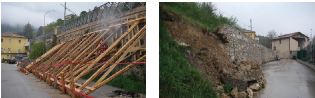
Figure 40. Examples of damage to masonry retaining walls.
