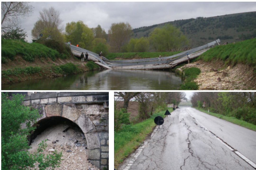
Figure 38. Collapse bridges and damaged road surfacing.
