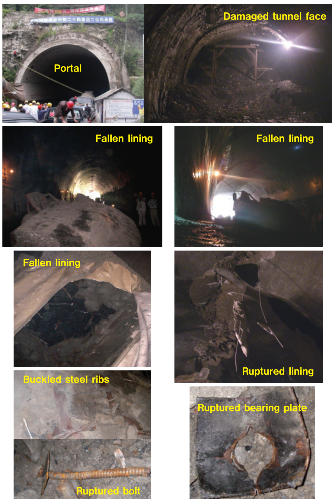
Figure 24. Views of damage at Jiujiaya Tunnel
