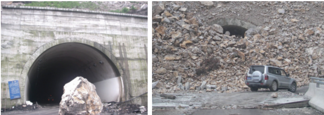
Figure 21. Damage to tunnel portals
