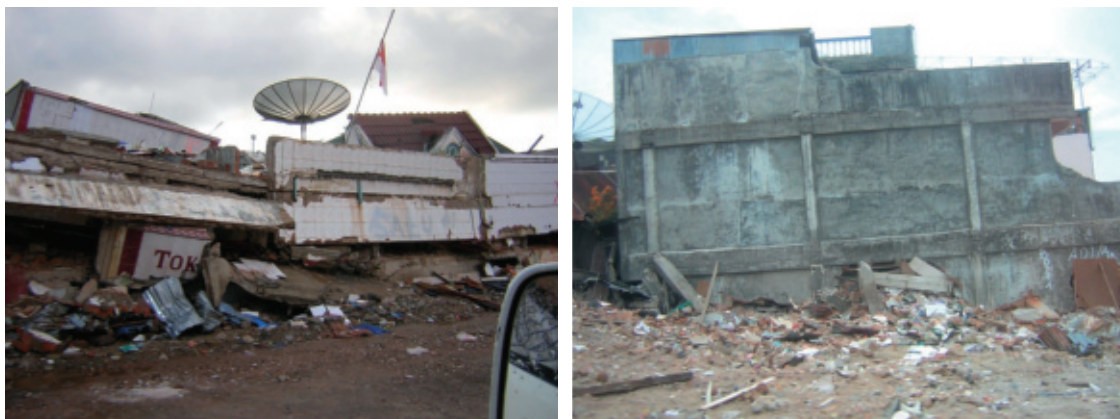
Figure 11 Failure of buildings due to soft floor effect
