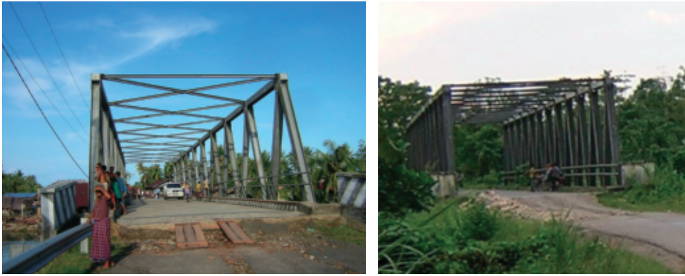
Figure 19 Settlement of approach embankments of bridges
