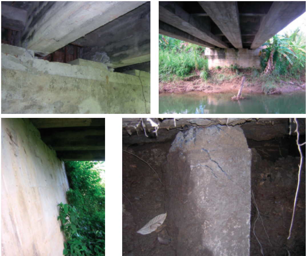
Figure 17 Some examples of damage to RC bridges
