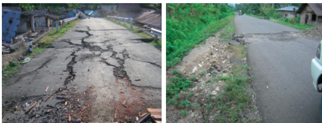
Figure 13 Damage to roadways
