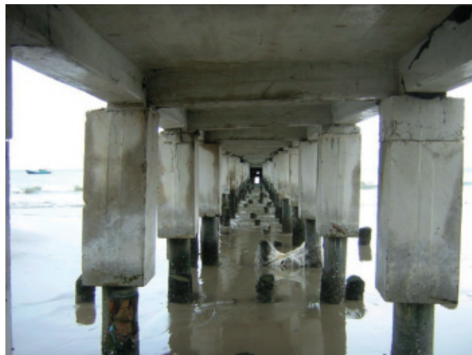
(a) Damage at Gunung Sutoli port
