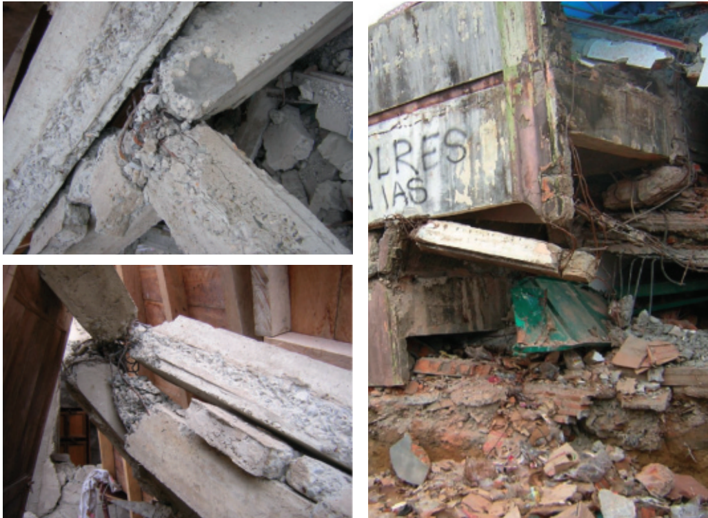
Figure 10 Typical poorly constructed column-beam joints
