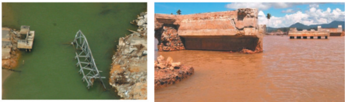
(a) Collapsed truss bridge (b) Collapsed concrete bridge
