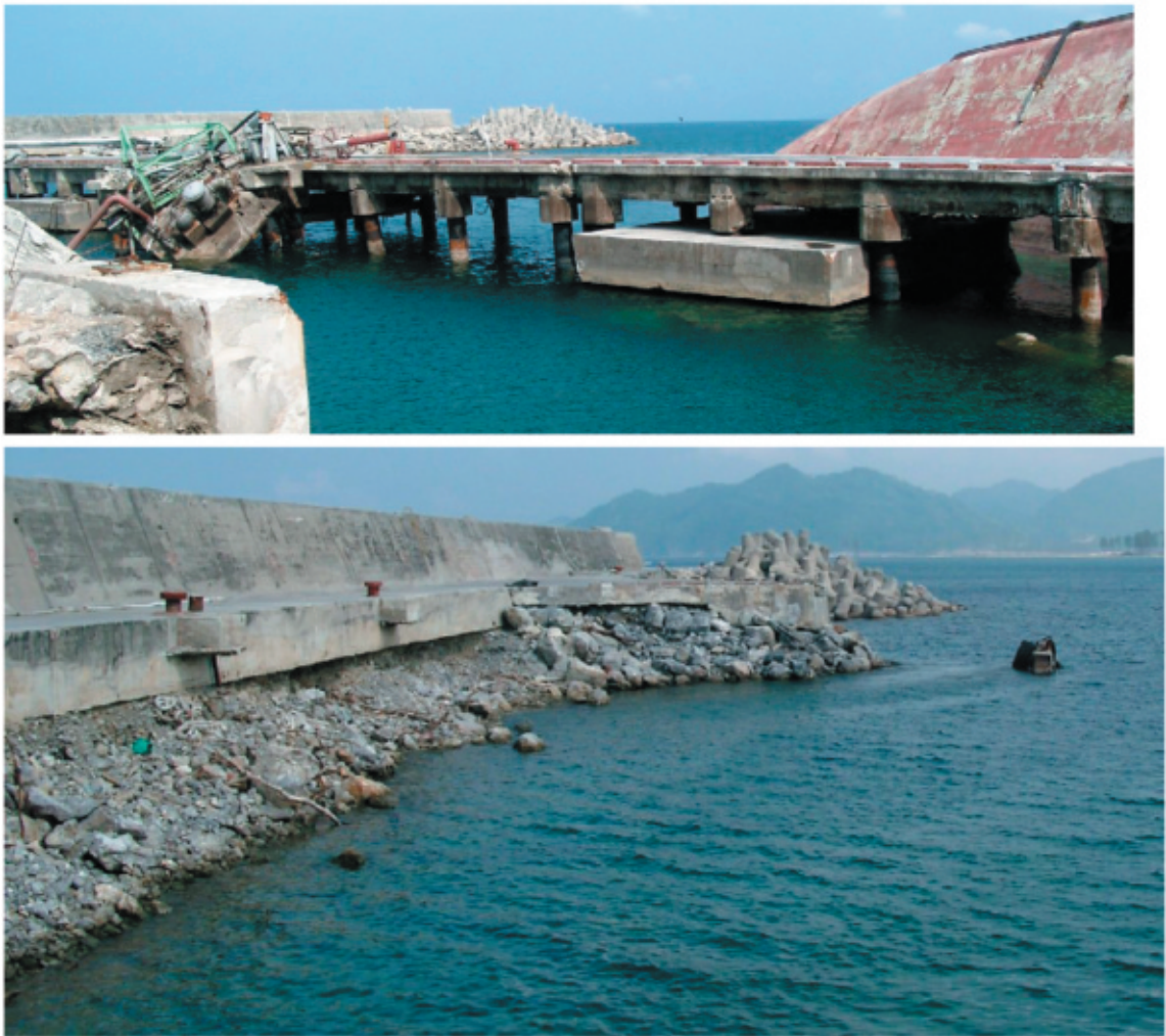
Figure 13 Damaged wharf and displaced tetrapods of wave-break at Lhonga port
