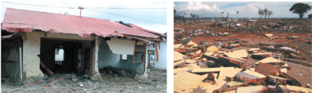
Figure 17 Damage to masonry (brick) buildings
