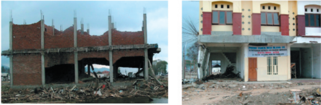
Figure 18 Damage to RC buildings in tsunami-affected area
